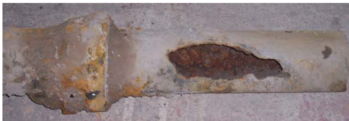
Above, is an example of deteriorating cast iron pipe, circa 1900. PICTURE: AQUA NEW JERSEY, INC.
