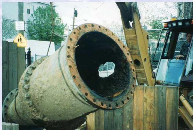
The above picture shows how a hole can be blown through an aging water main that has thinned through deterioration over time. PICTURE: UNITED WATER
