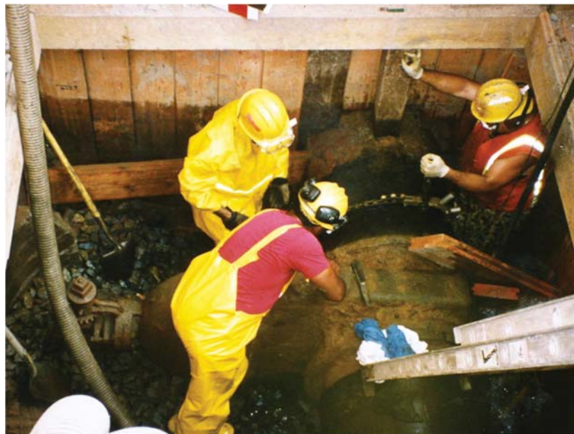
The inevitable impacts of not starting to address this problem now could result in increased service interruptions, and more frequent and costly emergency repairs such as this main break in New Jersey depicted above. PICTURE: UNITED WATER
