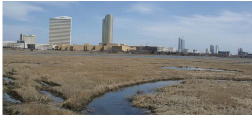
Above: Work will be performed on the sanitary force mains using horizontal directional drilling for a distance of approximately 2000 feet underground in the waterways of Penrose Canal and Clam Thorofare in Atlantic City. PHOTO: ATLANTIC CITY SEWERAGE COMPANY
